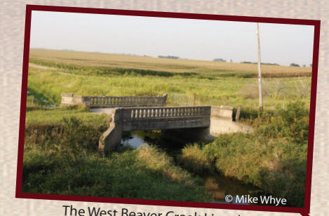
The West Beaver Creek Lincoln Highway Bridge was built in 1915, and despite being 100 years old, it is still in great shape.
